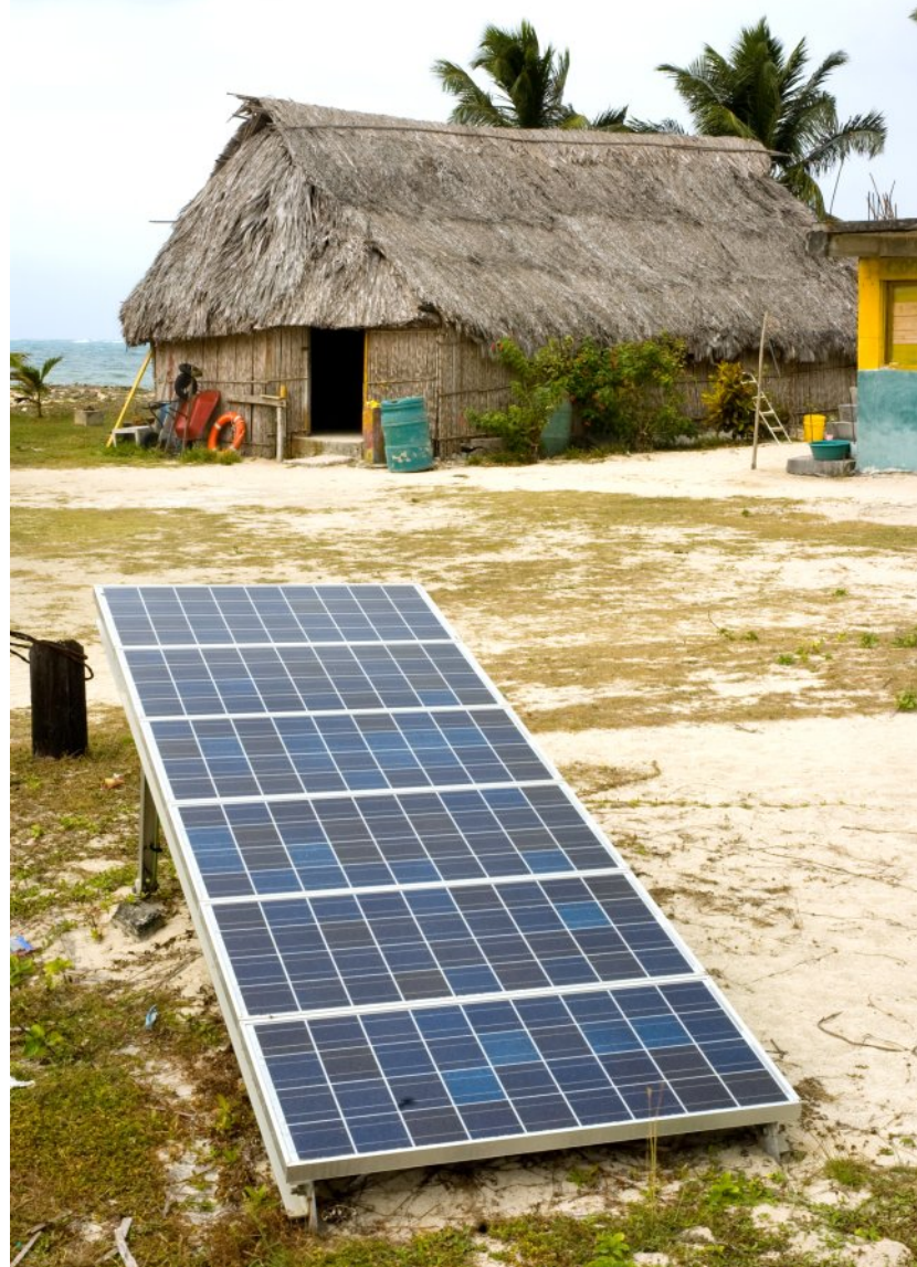
Solar power panel provides island power, Guna Yala, Panama. Ronnie Hall/CIC
